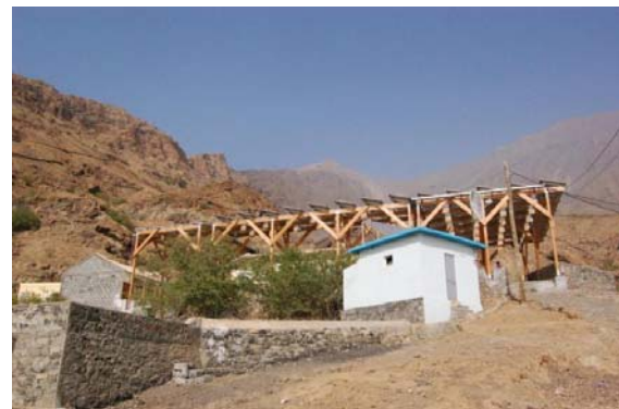
Figure 6: PV Pergola installed at the village's schoolyard (Photo: TTA)
